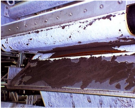
Wastewater solids slide from the Middlebury, VT belt filter press, ready to be treated to make biosolids.
